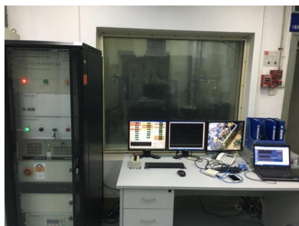
Fig. 4. Measurement and control system.
