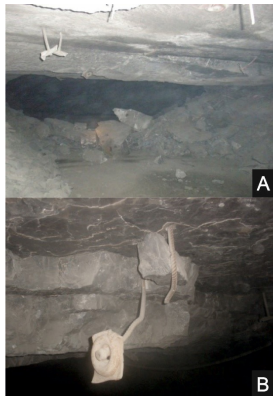
Fig. 1. Roof falls in one of the underground ore mines in the Legnica-Głogów Copper Belt; A) partial filled room by means of roof rocks, B) roof falls of stratificated roof layers.
