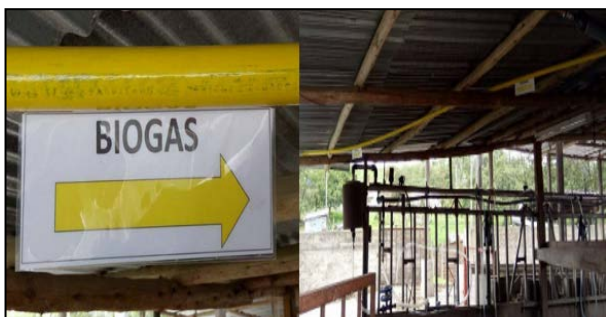
Figure 9. Transport of the biogas by means of a yellow polyethylene pipe.
