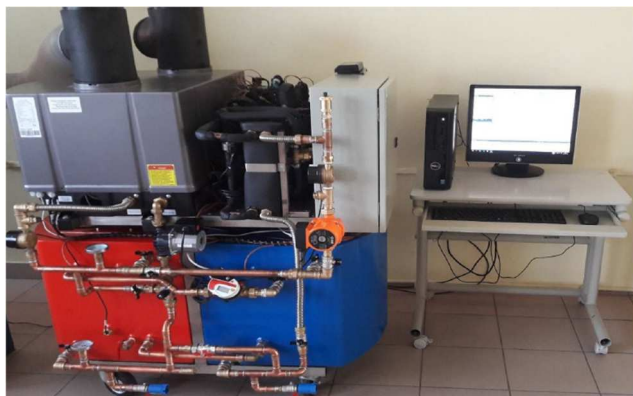
Fig. 2. Installation of a DHW heat pump in a research stand
