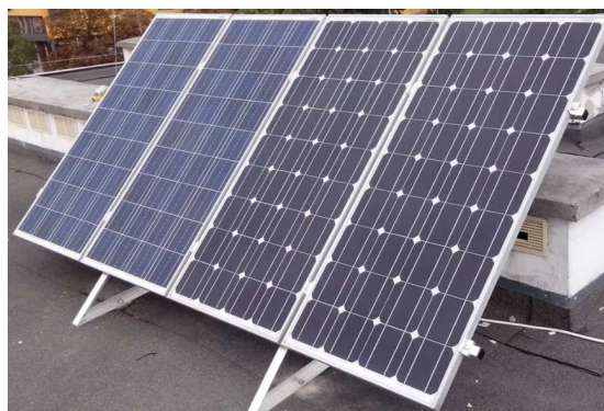
Fig. 1. Photovoltaic PV generator: left side polycrystalline PV modules - CL-130-12 model, and right side PV monocrystalline modules – AEMF 130 model
