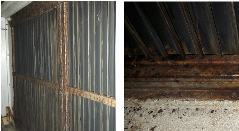
Fig. 6. View of the evaporator area in unit 1.
