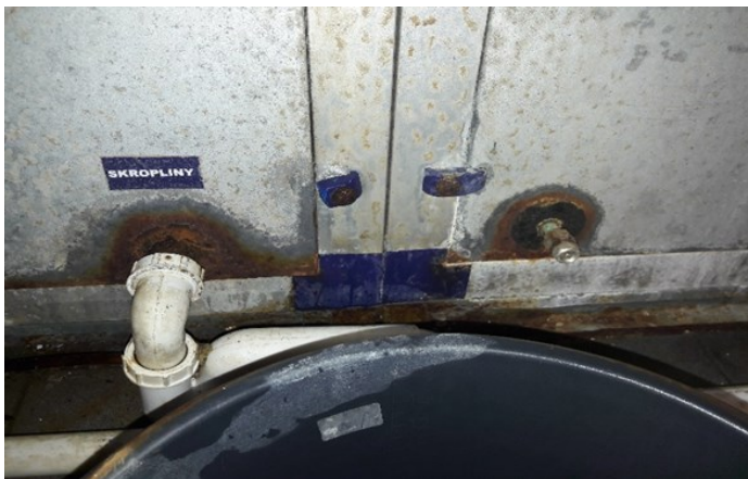
Fig. 2. View of the external cover panels of the air handling unit (air handling unit 2).
