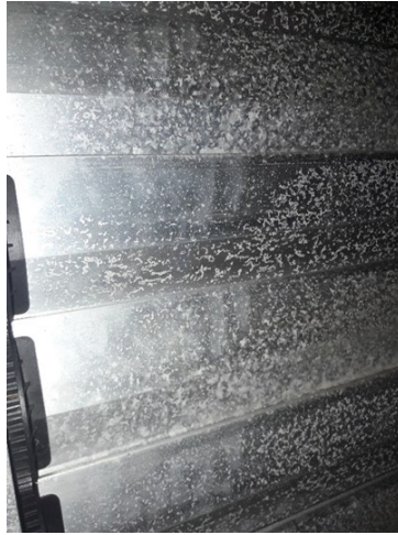
Fig. 5. View of the damper blades' surfaces made of aluminum in unit 1.
