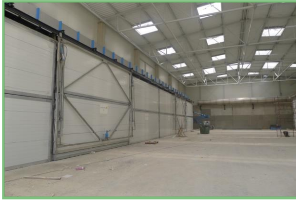
Fig. 1. Bioreactor – a biological waste drying chamber.
