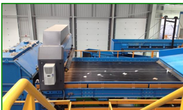
Fig. 4. Mechanical waste treatment station.
