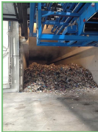
Fig. 2. Interior of a biological drying chamber.
