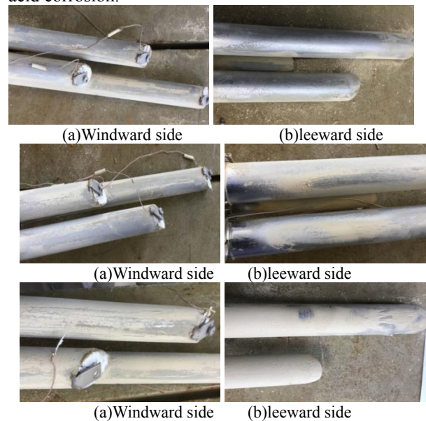
Figure4 Pipe wall gray area conditions in the temperature of 80°C/ 70°C/ 60°C
