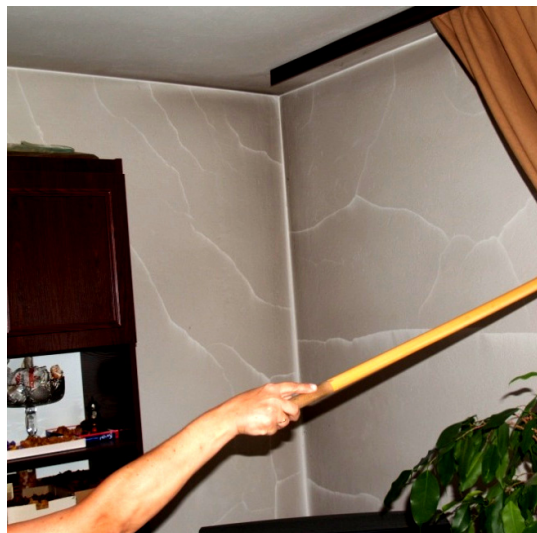
Fig. 1. Wall scratches in the area of the outer corner of the building
