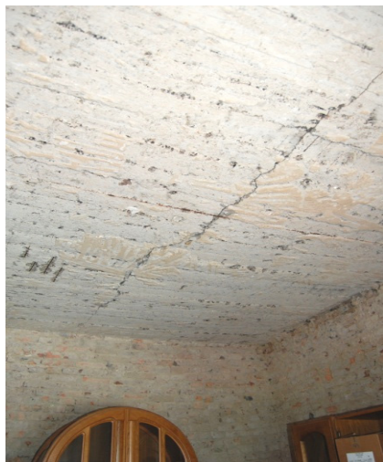
Fig. 7. Cracking of a reinforced concrete floor slab.
