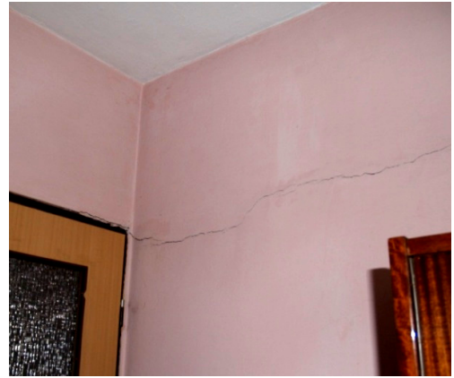
Fig. 6. Horizontal cracking of the concrete dilatation wall
