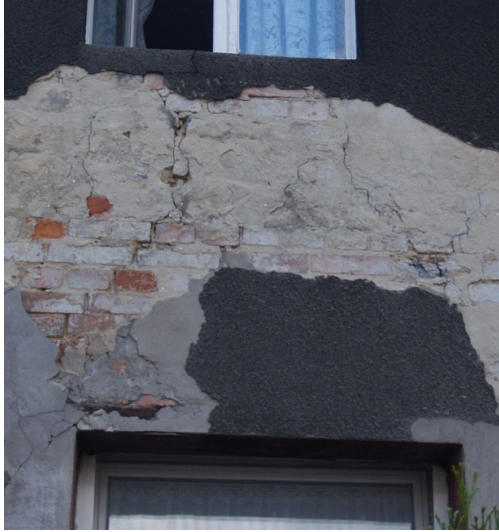
Fig. 3. Visible disintegration of the wall by the window
