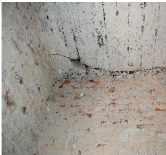
Fig. 8. Cracking of a reinforced concrete floor slab based on.
