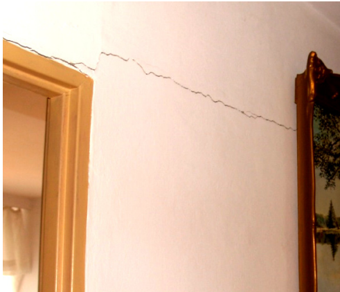
Fig. 5. Horizontal cracking of the concrete inner wall
