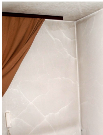
Fig. 2. Wall scratches in the area of the outer corner of the building
