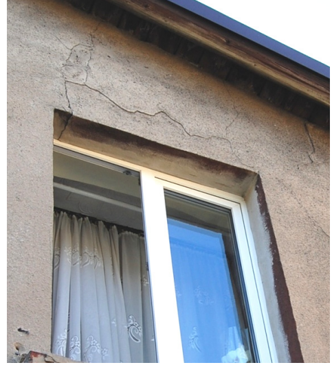
Fig. 4. Cracking and displacement of the lintel of the window
