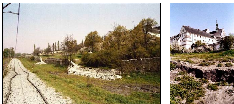
Fig. 3 Deformation of the track and destruction of the wall and cracking of the soil in the monastery's garden [4]
