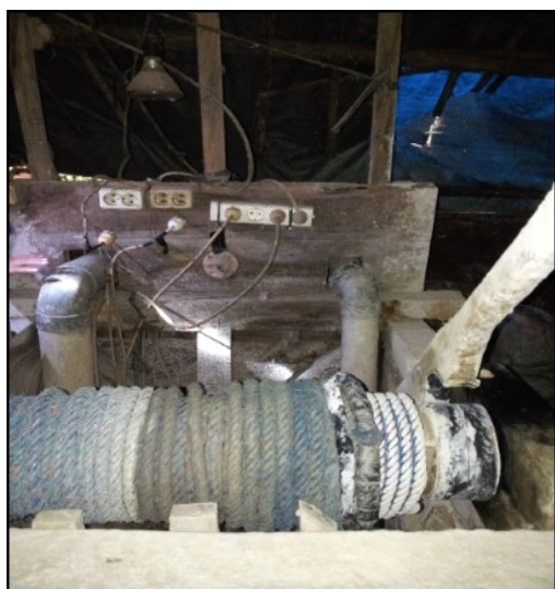
Fig. 2 Electricity and air lines to the site
