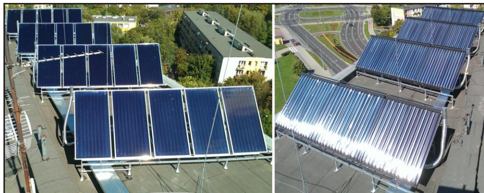
Fig. 1. Flat plate solar collectors connected in series of 5 units in one section (left side of the fig.), and evacuated tube solar collectors connected in series of 3 units in one section (right side of the fig.).
