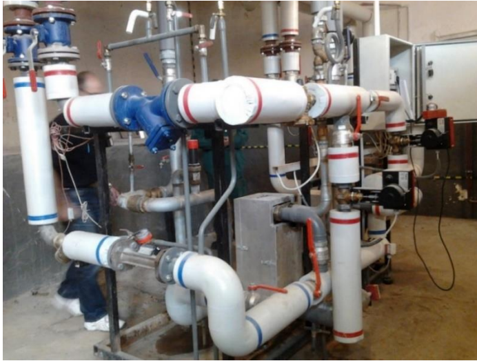
Photo 1. T15 Heating station.
