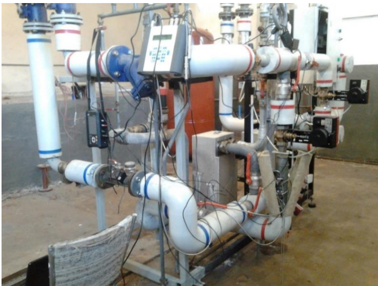
Photo 2. T16 Heating station.
