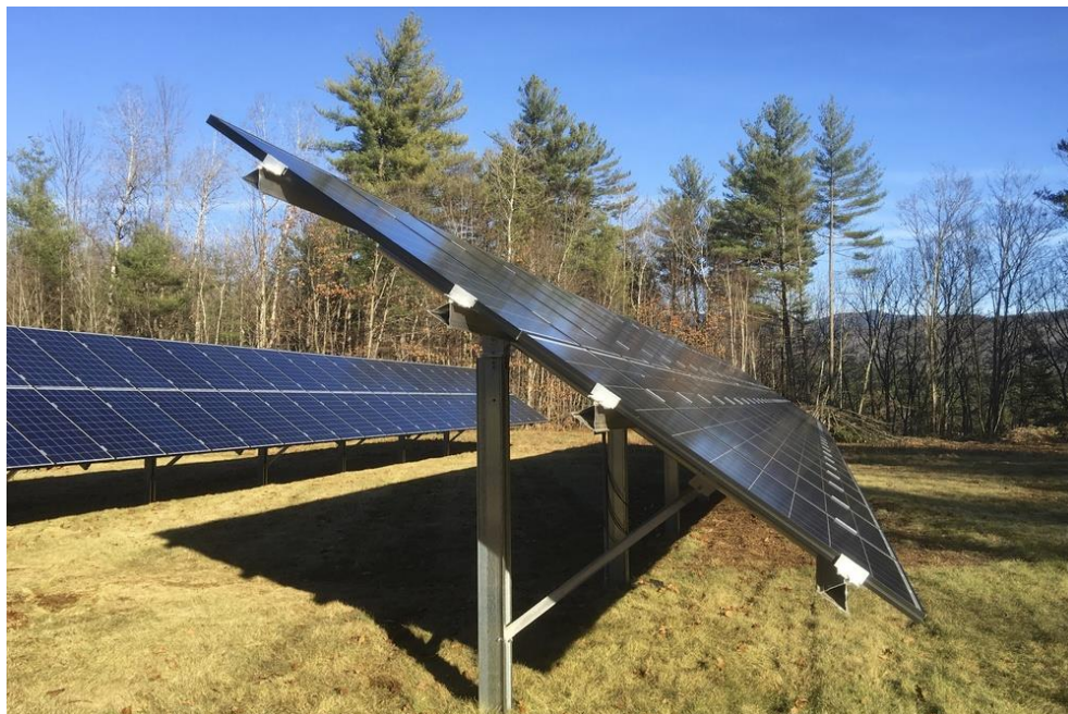
Fig. 1. Ground-mounted solar photovoltaic arrays at the Hubbard Brook Research Foundation. The system's estimated energy payback period of 2.4 years was significantly less than the simple payback period, 13.3 years. Note the driven-post system reaches soil depth of 2.4m, and requires no concrete to install.
