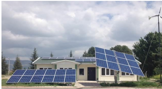
Fig 1. The Installed fixed (left side) and sun tracking solar PV panels (right side) with same capacity (3 kW) in Iki Eylul Campus of Anadolu University, Eskisehir, Turkey.
