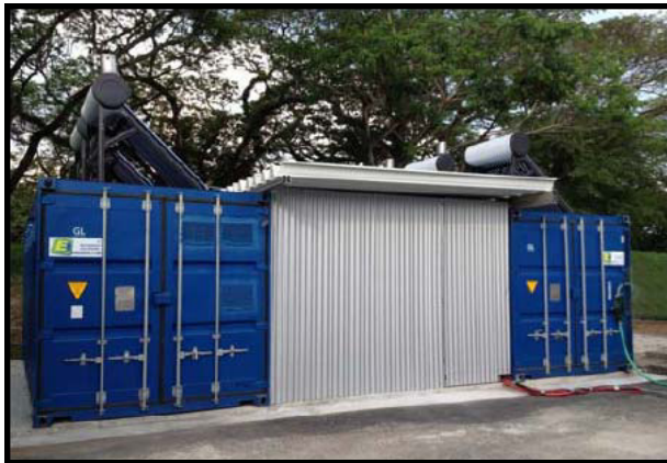
Figure 1: Prefabricated mini biogas power plant
