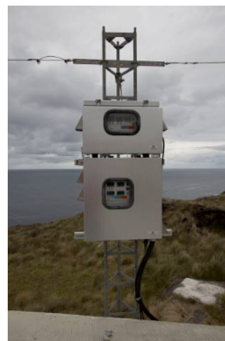
Figure 2. Tekran front-end modules 1130 and 1135 installed on the roof Pointe Bénédicte's laboratory at Amsterdam Island.
